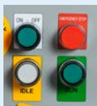
Control panel labelling
