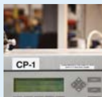
Control panel and electrical panel labels
