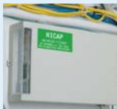
Control panel labelling
